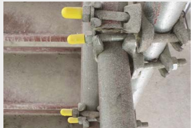
All scaffold bolts projecting into walkways and staircases need to be capped
